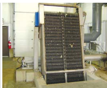
Waste Water Automatic Channel Screen
