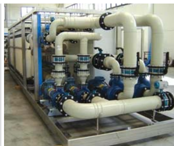
Ultra Filtration Plant 200 m 3 /h
