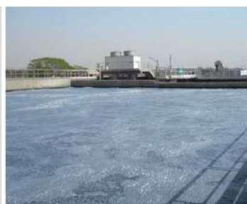
Waste Water Aeration Tank With Cooling Tower
