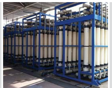
Ultra Filtration Plant 500 m 3 /h
