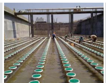
Waste Water Aeration System
