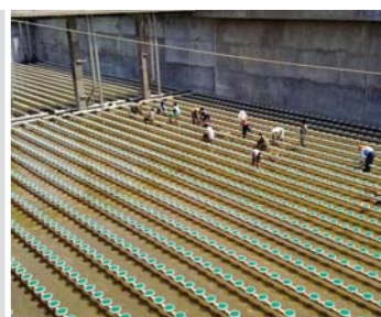
Waste Water Aeration System 500 m 3 /h India
