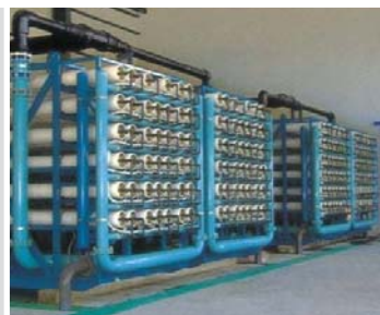
Seawater Treatment System
