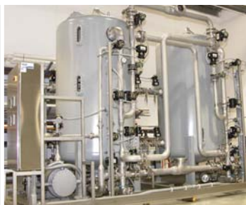
Demin Plant 30 m 3 /hr
