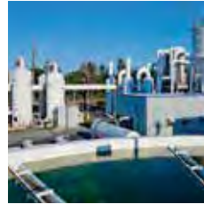
Water & Wastewater Treatment
